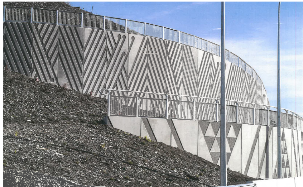
CONCRETE TILT SLAB WITH ENGRAVING - TE MOANA ROAD INTERCHANGE, PEKA PEKA HIGHWAY
